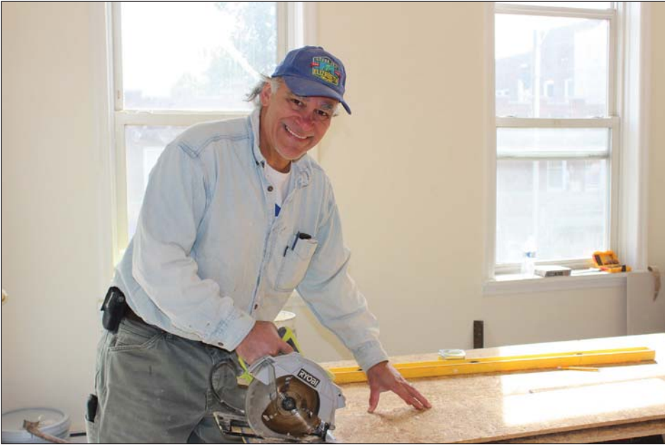
David Levenberg, Habitat for Humanity of Greater Newark volunteer, working on a Habitat Critical Repair project on Armstrong Avenue in Jersey City.
