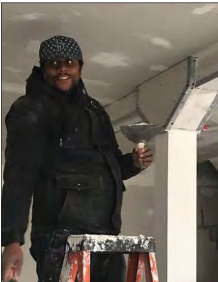
Alphonso Richards, Habitat of Greater Newark's Site Supervisor, plasters a ceiling this fall.
