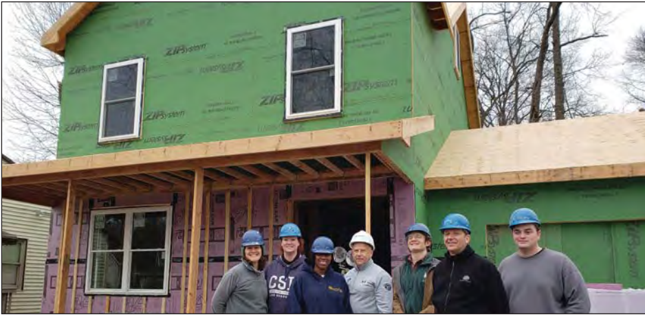
Volunteers from J.M. Huber Corporation pose in front of our build at 24 Burnet Street in Livingston this February.
