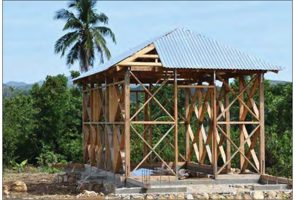
A home under construction in the southwest of Haiti. The wood beams provide more durability than a traditional Haitian home built using concrete blocks.
